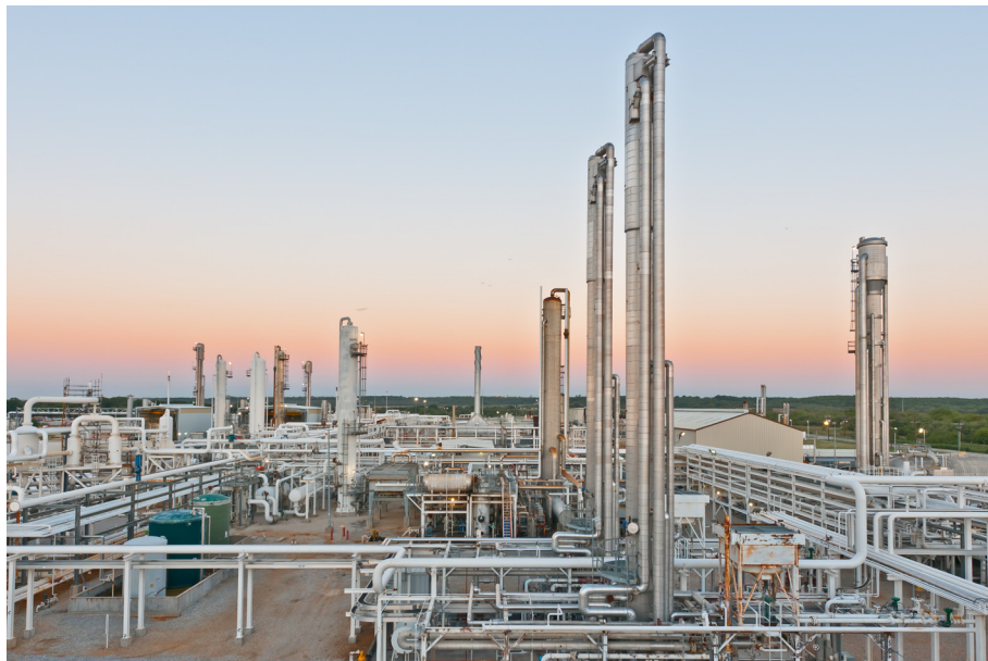
The Bridgeport gas processing plant located about 45 miles northwest of Fort Worth, Texas serves Barnett Shale production.
